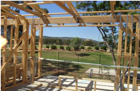
View from first floor resident room at Magill over looking the Hectorville Oval with the hills in the background.
